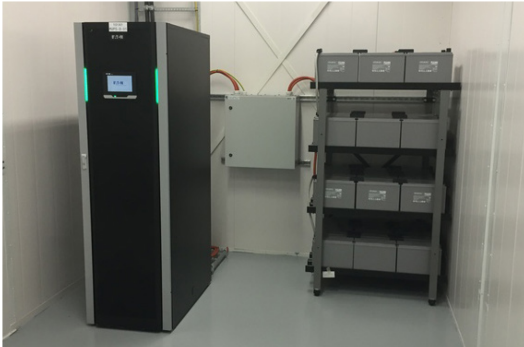
93PM and batteries
